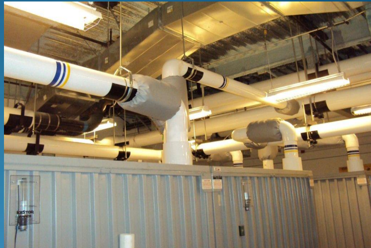
Pipe Valves and Duct work at PCAP
